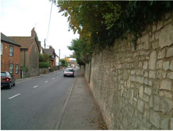
Trees overhang the retaining wall on the west side of High Street.
